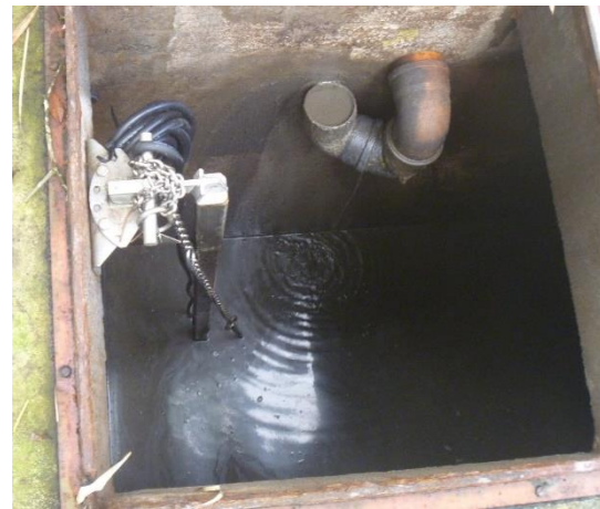
Figure 2.4 - Relevage des eaux brutes
